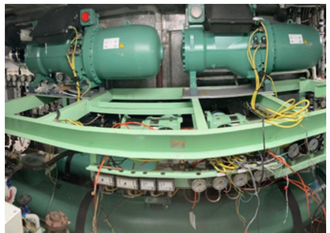
New chiller (compressor, evaporator, liquefier)
