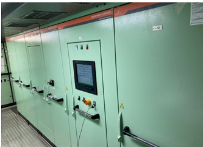
New frequency converter Pod drive portside
